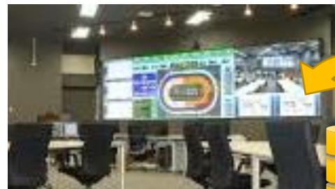
ITER REC Room
